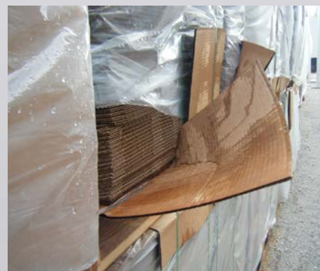
Conventional wrapping - Poor protection against rain, dust and contamination.
